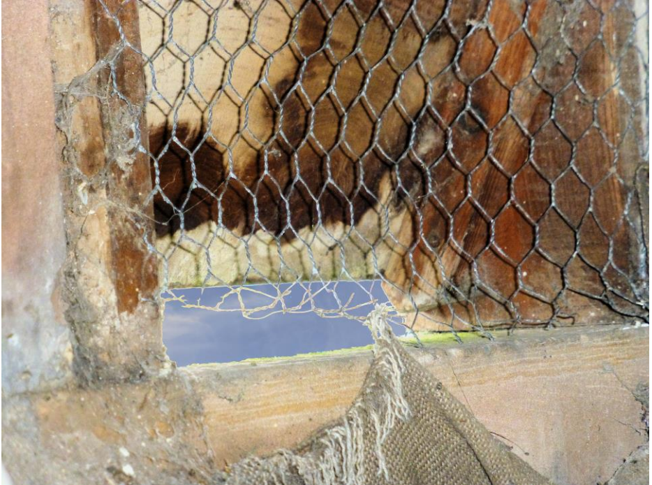
Canon Pyon Church Tower with its new opening allowing bats entry
