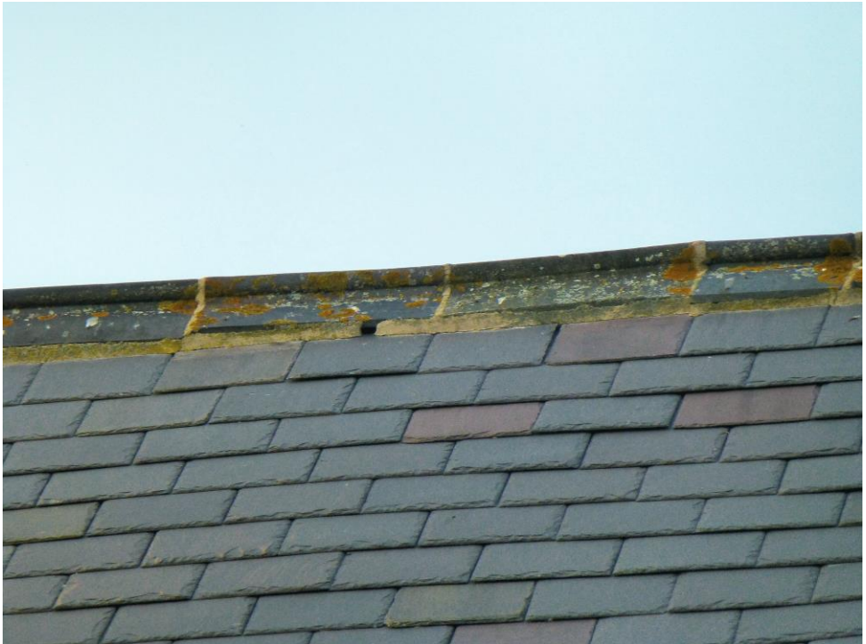
Purpose-made gap under a ridge tile allowing access for crevice dwelling bats
